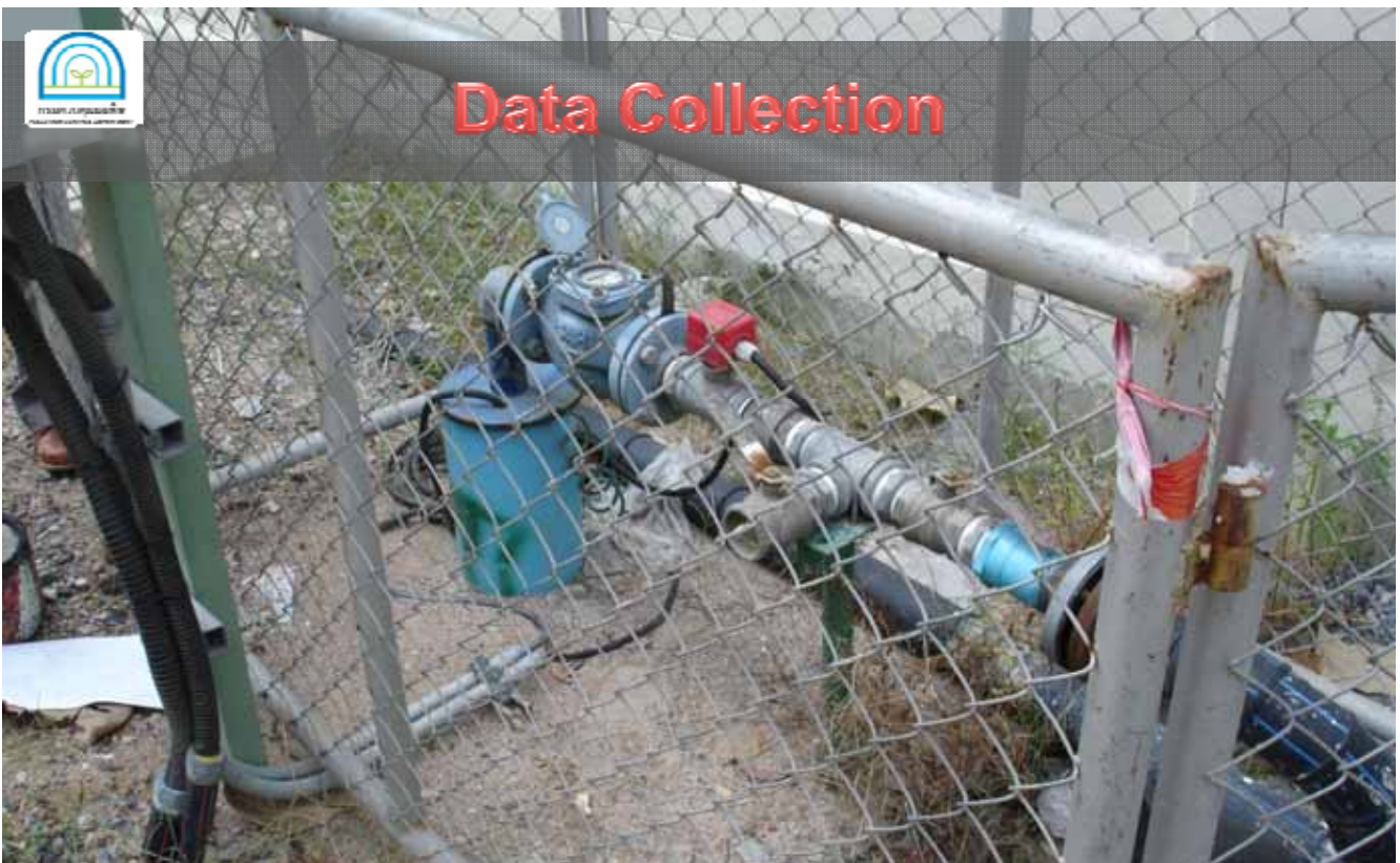
Ground water production well around 100 m depth
