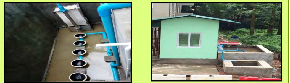
Location – YCDC Officer Housing-Membrane Bio-Reactor System (30m 3 /day, 38m 3 /day)
