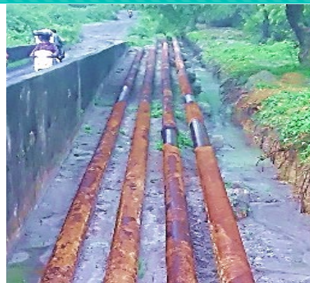
Water loss due to ageing infrastructure
